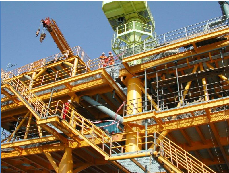
Above: Offshore operations, offshore platform.
